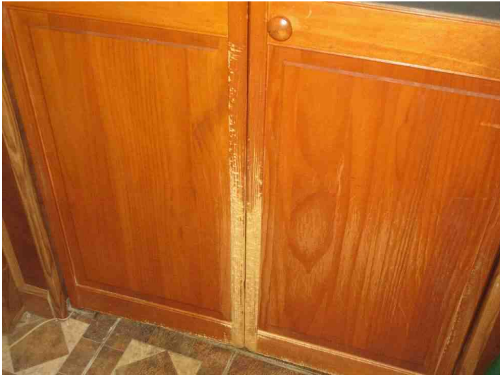
worn kitchen cabinets
