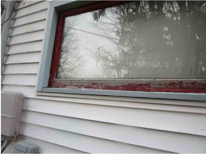
Windows (chipping/peeling paint detail)
