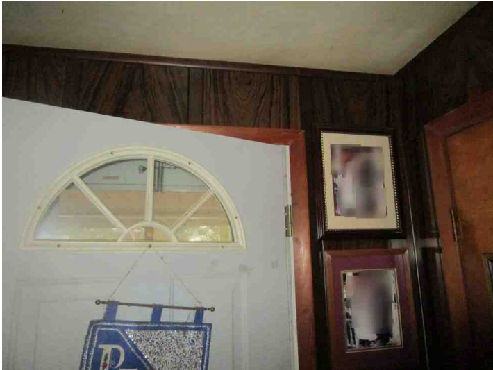
Foyer ceiling water stains
