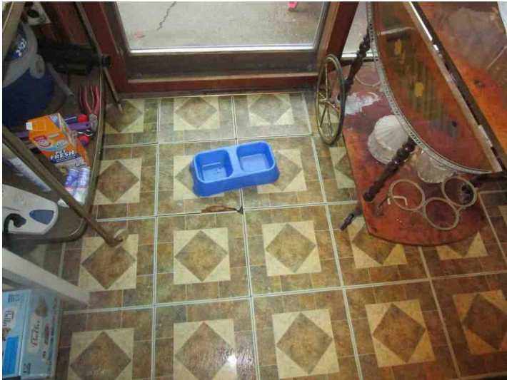
Laundry Room (floor detail) end of usefull life
