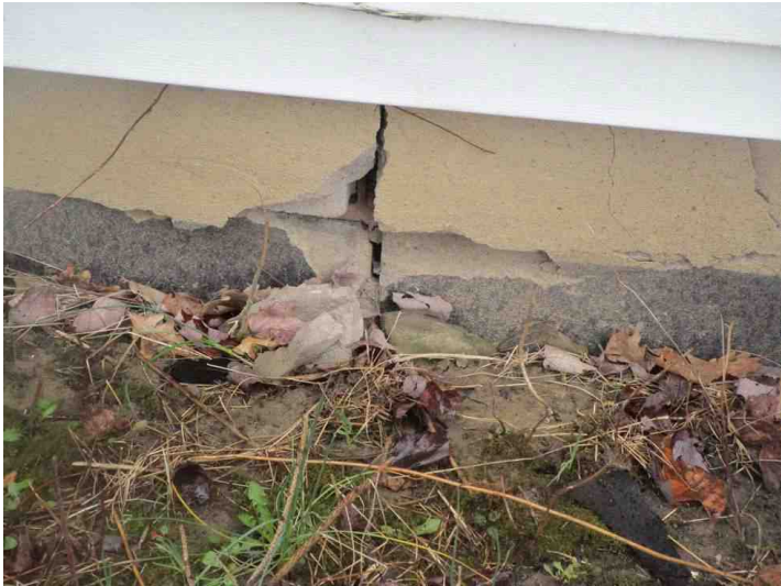
Foundation (settlement detail)
