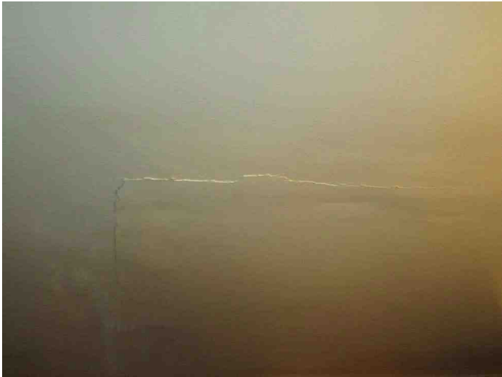
ceiling poor repair
