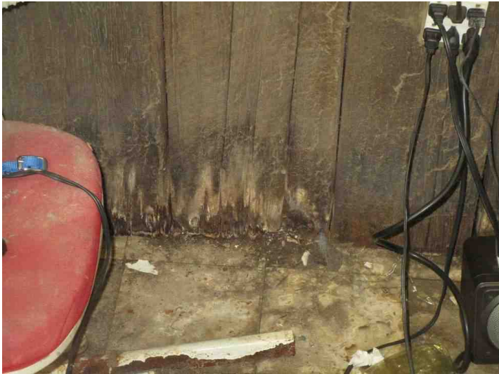
Basement (water damage detail)
