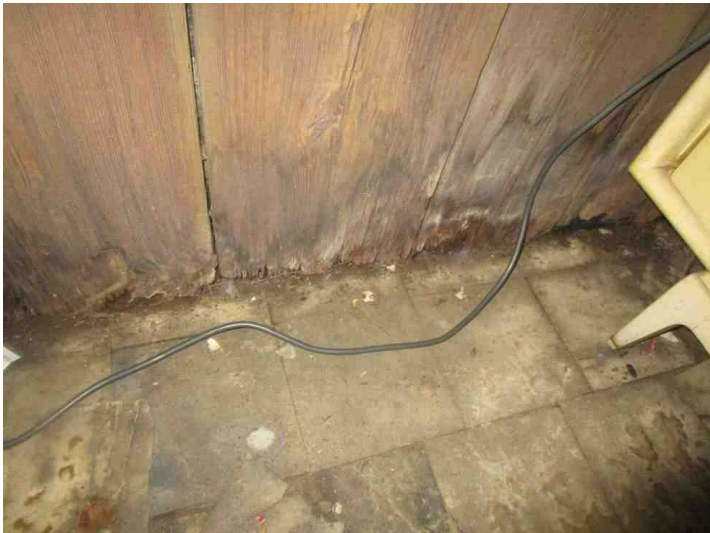
Basement (water damage detail)
