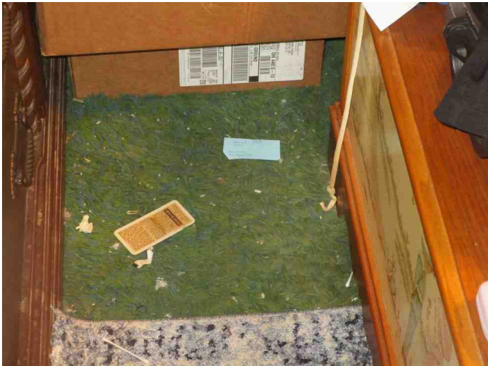
Bedroom 3 (floor detail) end of useful life
