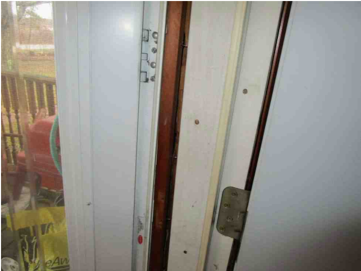
Door Jamb detail does not close correctly
