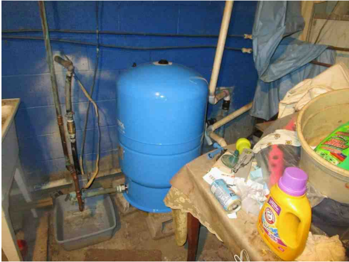
Water treatment system
