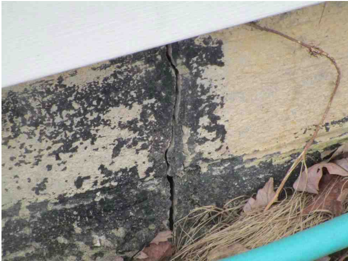
Foundation (settlement detail)
