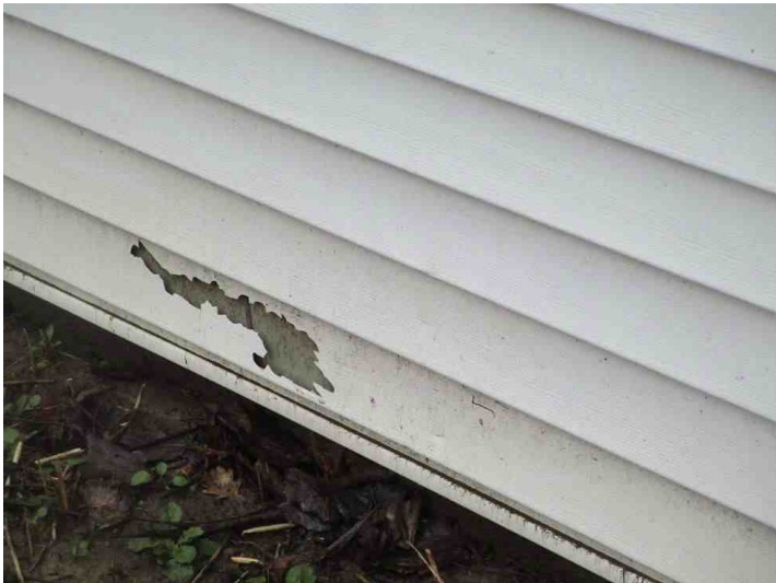
Vinyl Siding (damage detail)
