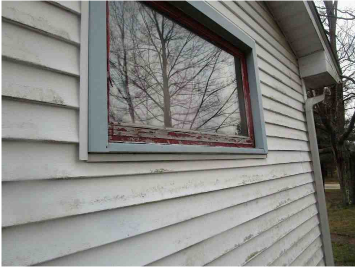
Windows (chipping/peeling paint detail)
