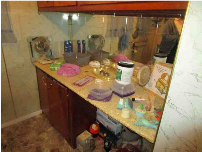
Bathroom worn cabinets
