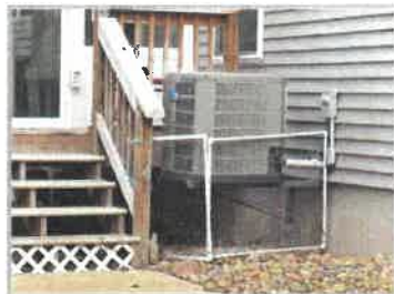
Central Air Unit
