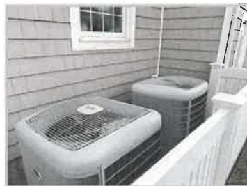
Central Air Unit
