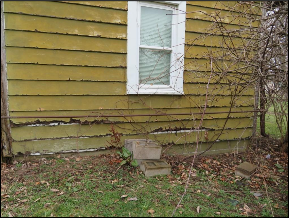
Deteriorating masonite siding on rear side of dwelling
