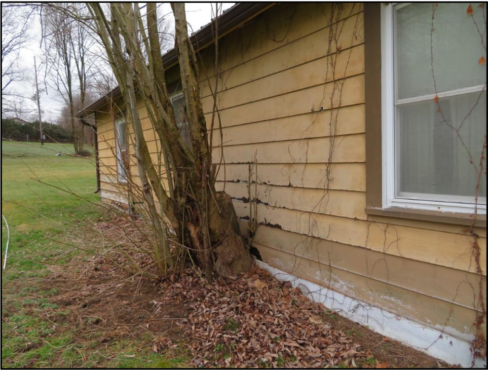
Tree growing into foundation on rear side of dwelling
