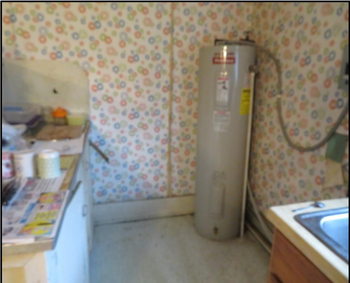
Hot water tank in kitchen
