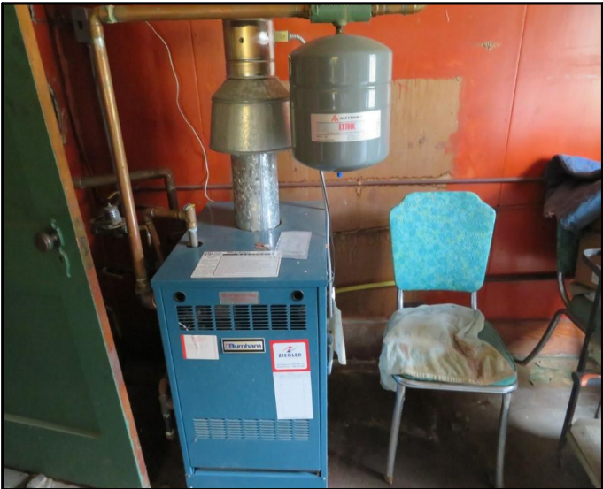
Hot water boiler in utility room
