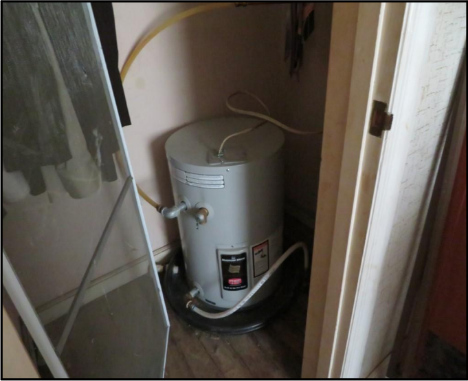
Hot water tank for hall bath in bedroom closet
