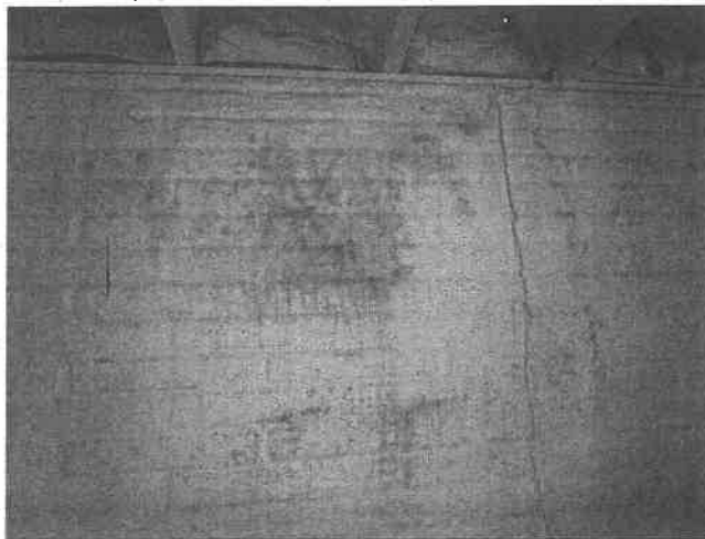
Basement (Settlement/Water Damage)
