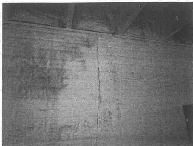
Basement (Settlement/Water Damage)
