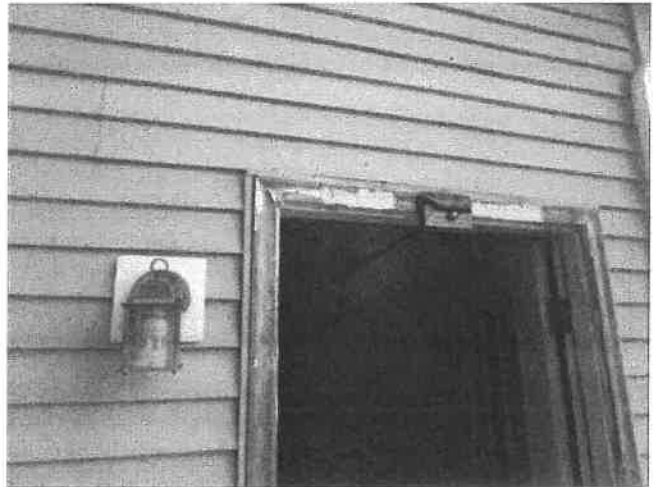
PEELING PAINT (Man Door)
