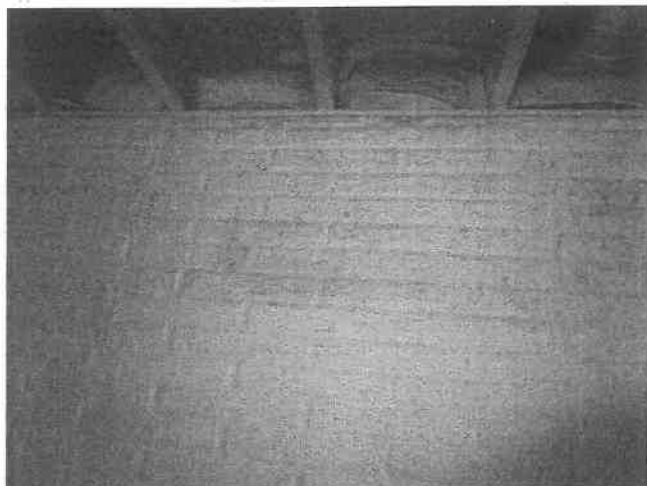
Basement (Water Damage)
