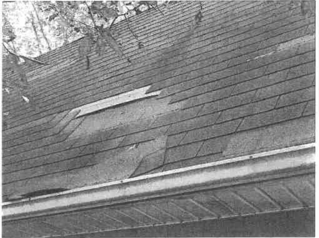
Barn (MISSING ROOF SHINGLES)
