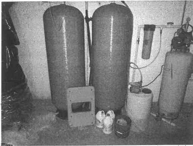
Water Treatment System
