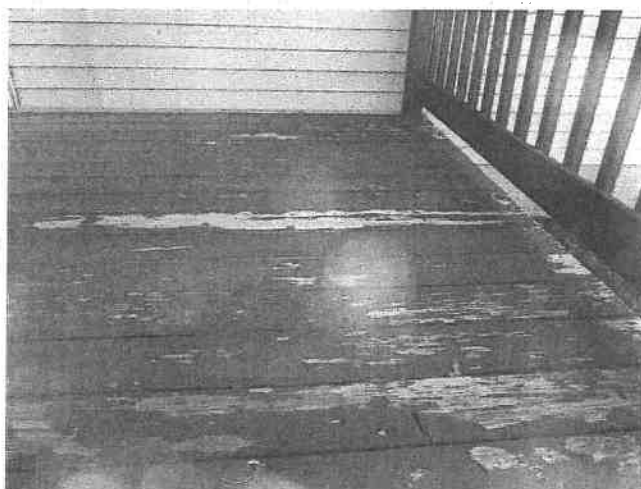
PEELING PAINT (Front Porch)
