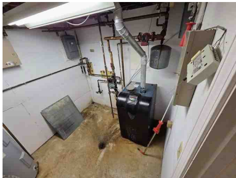
Water Boiler/Breaker Box
