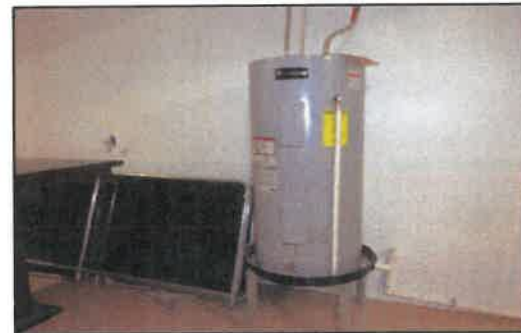
Hot Water Tank
