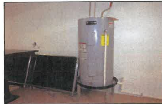
Hot Water Tank
